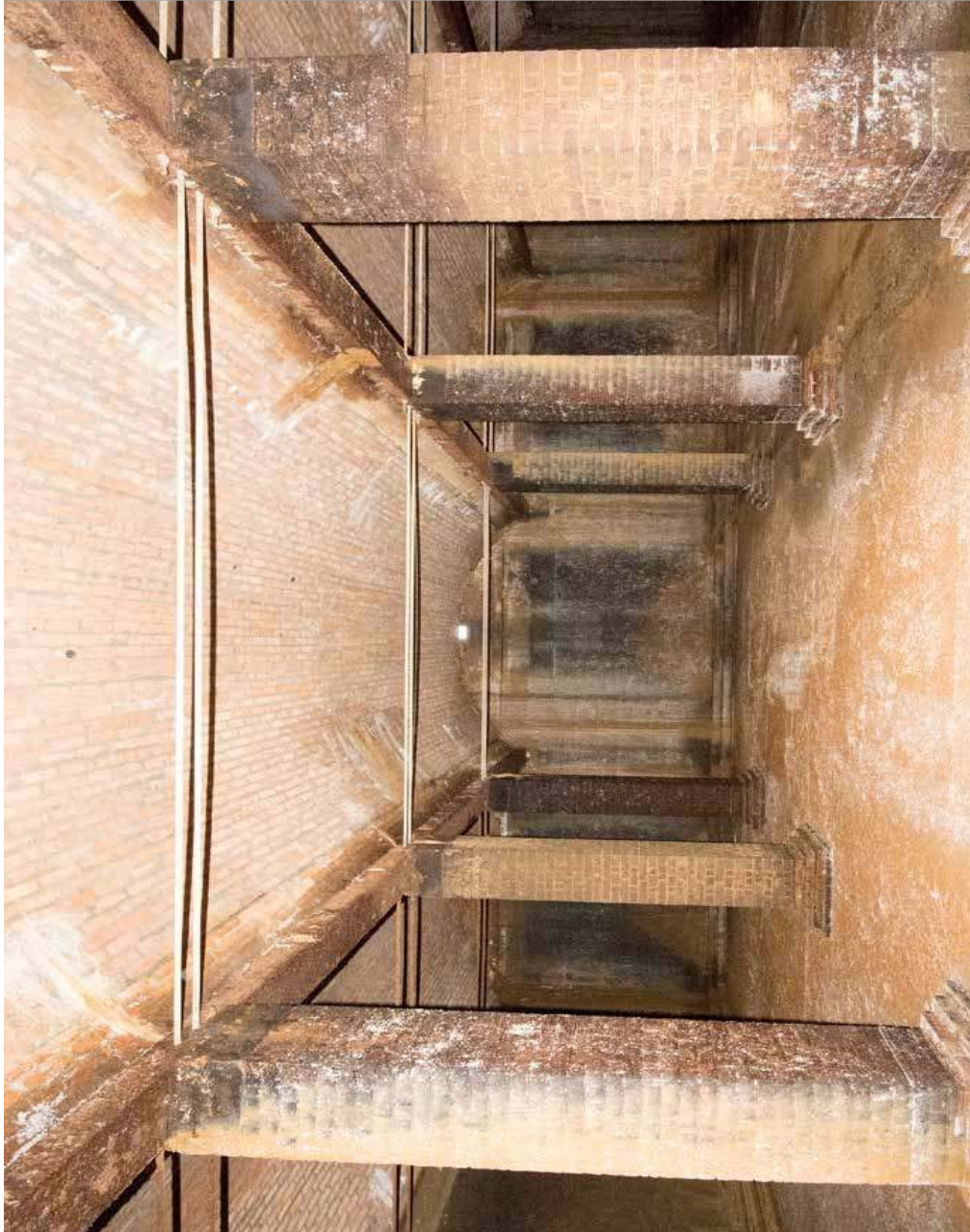
No. 1 Reservoir, 1882., Brown St Newcastle. Cast iron beams made in Rodger Bros foundry.
